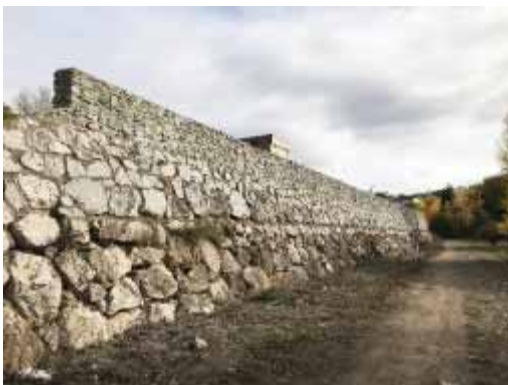
Raised 200 m-long wall at the confluence of two rivers where floods had occurred in the past (Spain)
